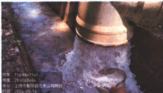
矿井水排放口DW001
